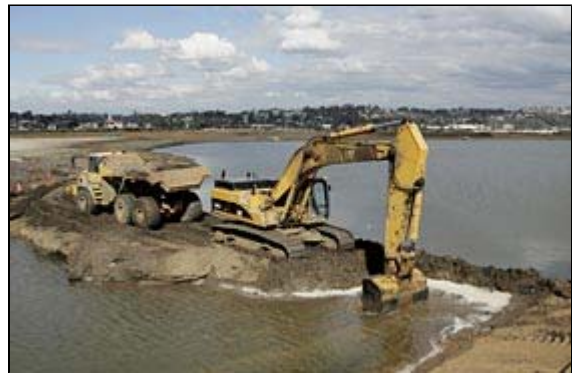
EDUARDO CONTRERAS / Union-Tribune Works crews removed the earthen dam at the mouth of the tidal basin yesterday, which then was connected to a channel of the San Dieguito River, which flows northwest to the ocean.
