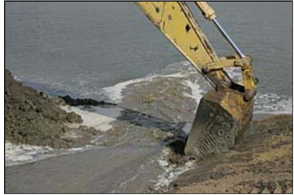
EDUARDO CONTRERAS / Union-Tribune A newly dredged tidal basin, which once was a Navy dirigible landing field, was connected to an ocean-going river channel – a key advance in the San Dieguito Wetlands Restoration Project under way on both sides of I-5 near the Del Mar Fairgrounds.
