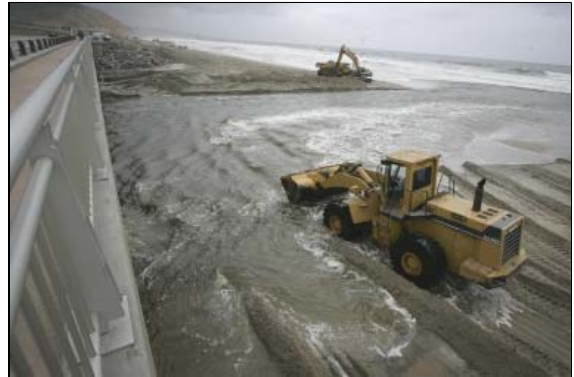
JOHN GIBBONS / Union-Tribune Heavy equipment works unplugging the mouths of San Dieguito and Los Peñasquitos lagoons near Del Mar, which closed six weeks ago after winter surf and currents blocked the openings with sand and cobbles.
