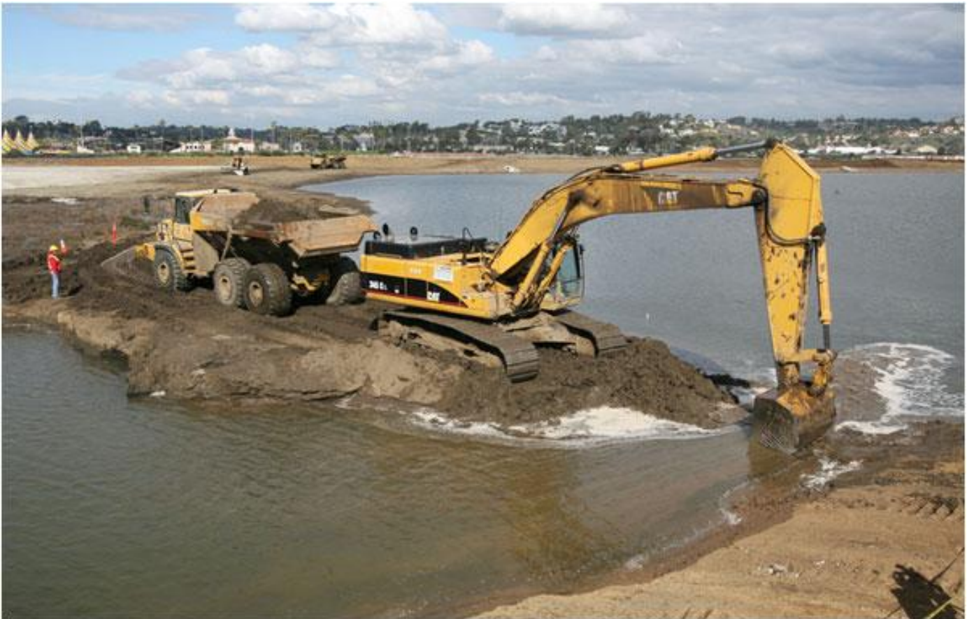
An excavator clears away a berm so that ocean water can flow into a man-made basin within the San Dieguito Lagoon in Del Mar on Wednesday.
