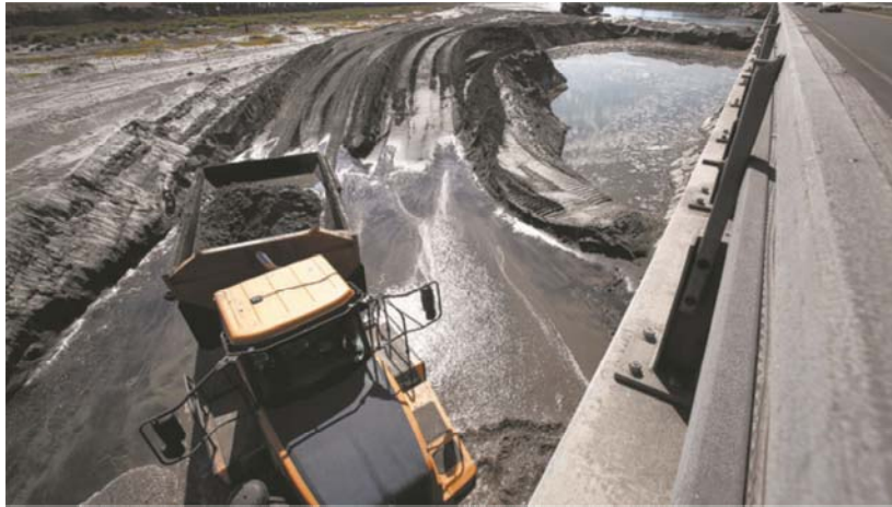
Construction crews are removing sand to open the mouth of San Dieguito Lagoon in Del Mar. — Peggy Peattie
